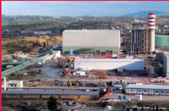
Structural Strengthening of new plant of High voltage Unit of DEI, Evia, Greece
